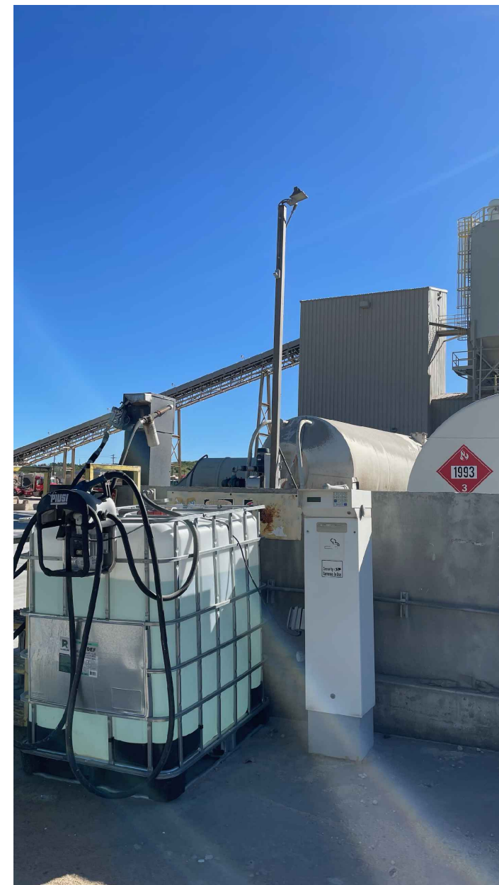
EXISTING FUEL TANKS IN CONTAINMENT FACING EAST
