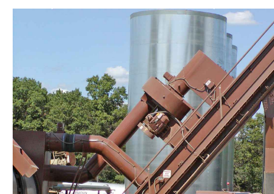
BLUE SMOKE FAN Notes: Part of blue smoke capture system. Captures emissions from asphalt mixing and silo loading process and returns them to be used as fuel.
