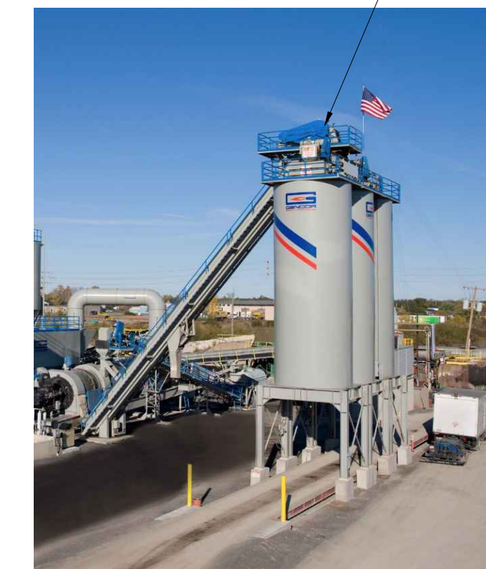
PRODUCT SILO Notes: Three product silos over single loading lane (see site plan and elevations) Painted Silo: Beige Support legs and structure: Beige Height: 50' to top of silo 70' - 4" top of conveyor and blue smoke capture system equipment Width: 15' - 11" Length: 43' - 11"
