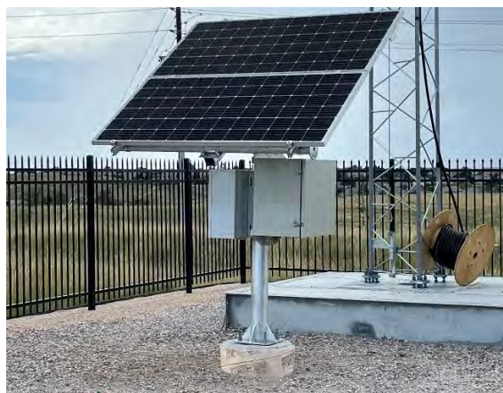
Figure 2: AMI Controls and Solar Panel
